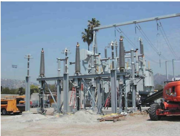
Figure 1 230-kV cable system installed in Los Angeles
