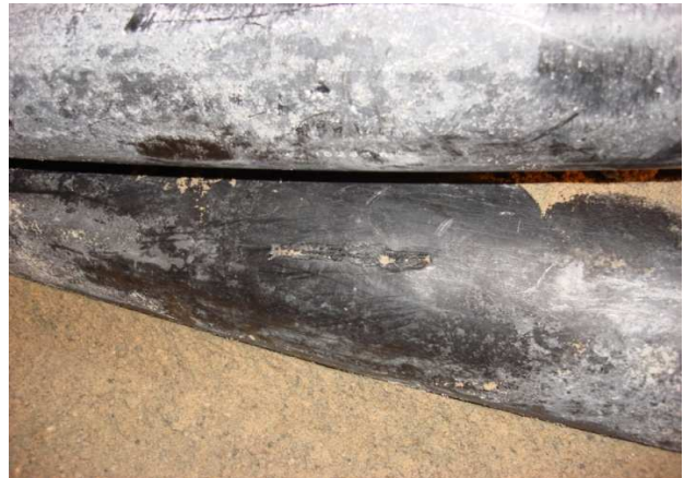
Fig. 2 Damage on a 380kV-Fluidfill cable
