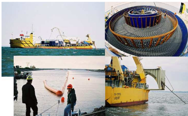
Fig. 1. Cross Sound project USA, 150 kV, commissioned 2002.
