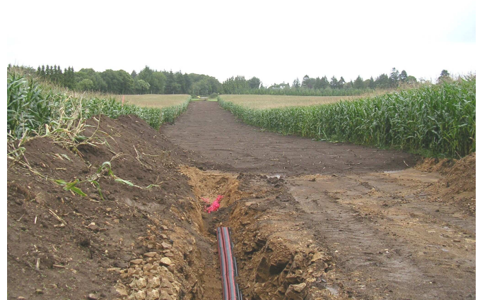
Figure 1 : Settlement of an underground power link straight across a field in western France.
