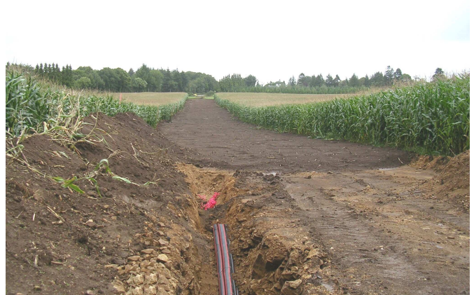
Figure 1 : Settlement of an underground power link straight across a field in western France.
