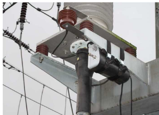
Fig. 1: Installed sensor and pre-amplifier.
