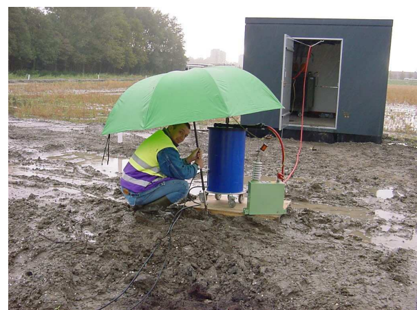
Fig 2: Example of on-site PD testing of 10kV XLPE insulated cable (tested in section) using damped AC voltages.
