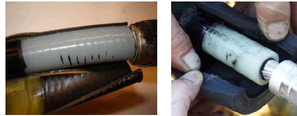
Fig 1: Example of wrong installation work (left) and insulation degradation (right) in a cable accessories. In all these types of insulation defects partial discharges are symptoms.
