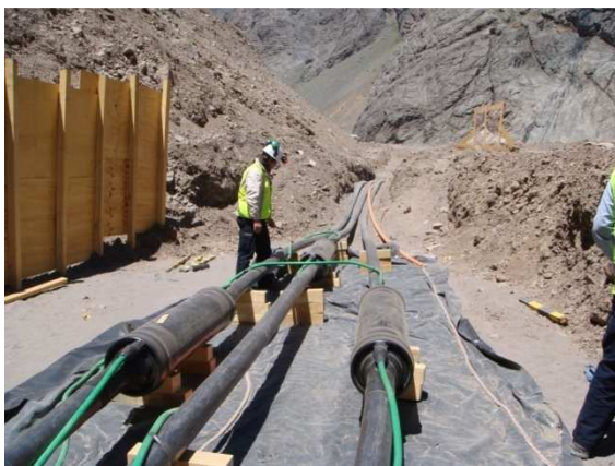
Figure 1 – 8 km of 220 kV XLPE Insulated Cable in Chile
