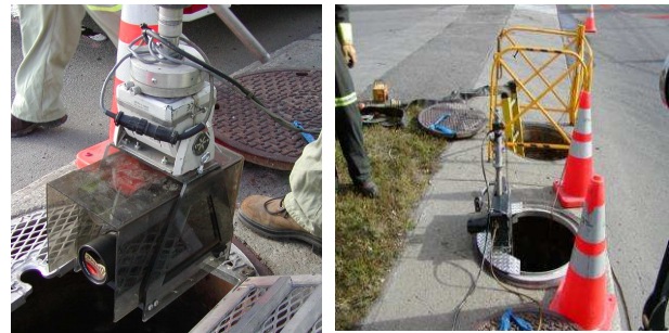
Figure 1. Left: housing with pan and tilt; right: pole placed into manhole
