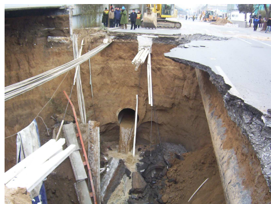
Figure 3. Photo of the cable tunnel collapse scene
