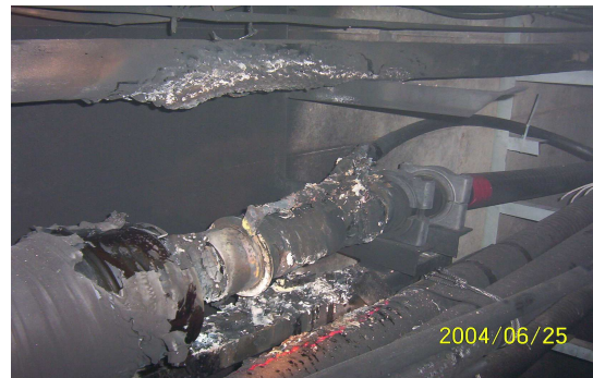
Figure 2. Photo of the cable malfunction accident
