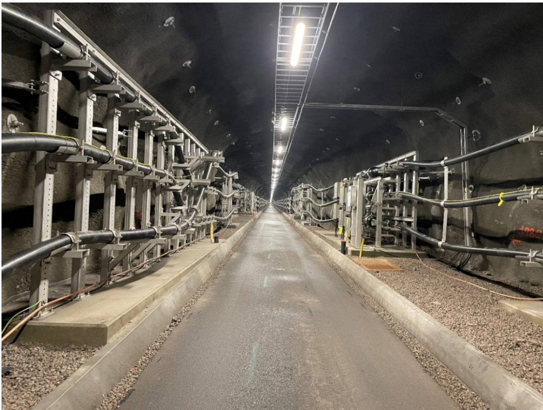
Fig. 1: View on the drill-and-blast tunnel with the two 420 kV circuits. On the left: cable phase transposition, on the right: joint support frame.
