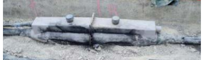
Fig. 2. 2021 failed blue phase joint. (Failed blue phase is the top joint in the photo.)
