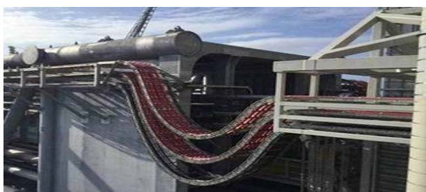
Fig. 01: Flexible tray [A bridge for cables connecting onshore and Offshore platforms]
