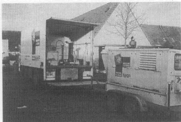
Figure 1: PD on-site diagnostic of a 10 kV power cable using 55 kV AC series resonance test set and an advanced PD analyzer TE 571.
