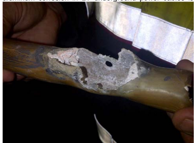
Fig. 1: Example of a cable section affected by aluminum corrosion. Unattached aluminum hydroxide is removed to show the extent of aluminum removal by the process.
