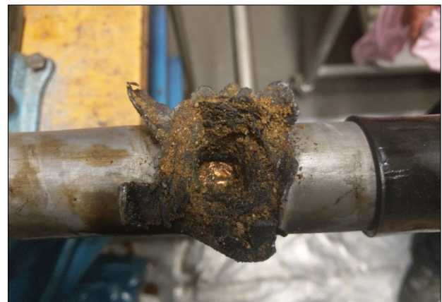
Fig. 2: elec. breakdown of an external gas pressure cable strand due to preceding PD-events at 2 \cdot U_0
