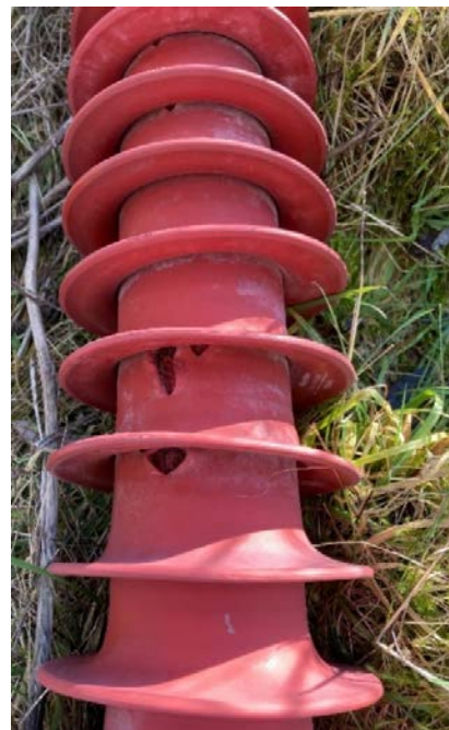
Figure 1: Example of visual defect at the cable terminations
