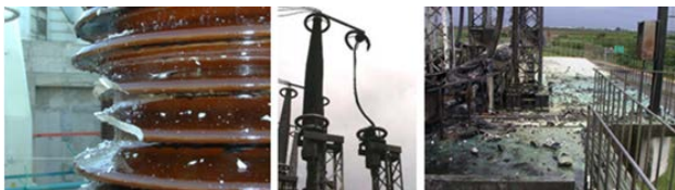
Fig. 1: Hazard area after accidents of liquid filled OSE
