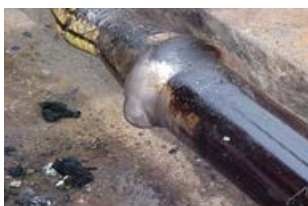
Figure 1 Typical leak on FFLP cable
