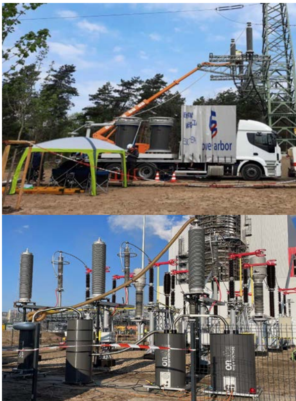
Fig. 1: Examples of AC Resonance System (ACRT) (top) and Damped AC Voltage (DAC) system applications for on-site testing of long, high-voltage cable systems (bottom) stresses that are higher than the dielectric strength of the
