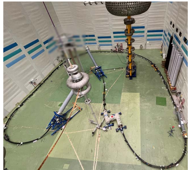
Figure 3: Cable connection assembly test setup for ±525 kV PQ test
