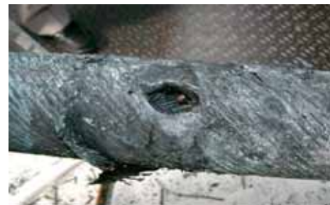
Figure 2: Cable breakdown in a tunnel duct
