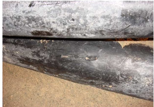
Fig. 2 Damage on a 380kV-Fluidfill cable
