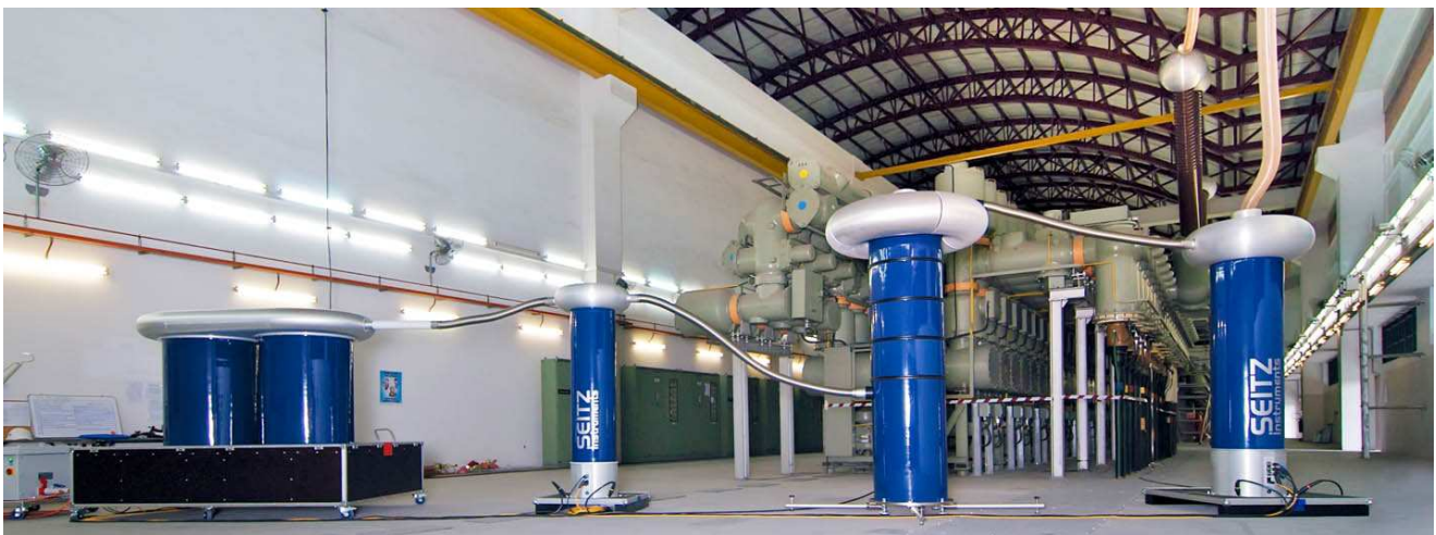
Fig. 1: On-site application of a 350 kV damped AC test system (OWTS HV Technology) on a 28 km long 230kV power cable connected with a test adapter to the GIS enclosed cable termination. The system consists of: (from the left to right) unit 1: High Voltage power supply Unit, unit 2: HV switch with light triggered thyristors (LTT), unit 3: Inductance Unit, unit 4: coupling capacitor, embedded computer system with remote control (Control unit, PD analyzer), Voltage Divider
