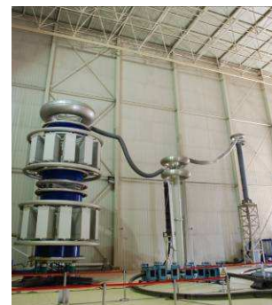
Figure 1 The 800 kV/30 A corona free series resonant test system at power frequency
