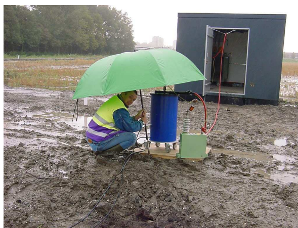
Fig 2: Example of on-site PD testing of 10kV XLPE insulated cable (tested in section) using damped AC voltages.
