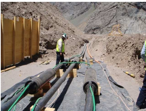
Figure 1 – 8 km of 220 kV XLPE Insulated Cable in Chile
