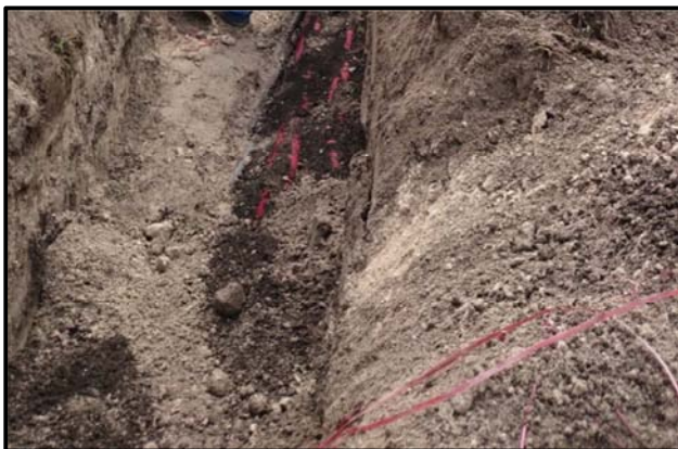
Fig. 1: Direct buried cables
