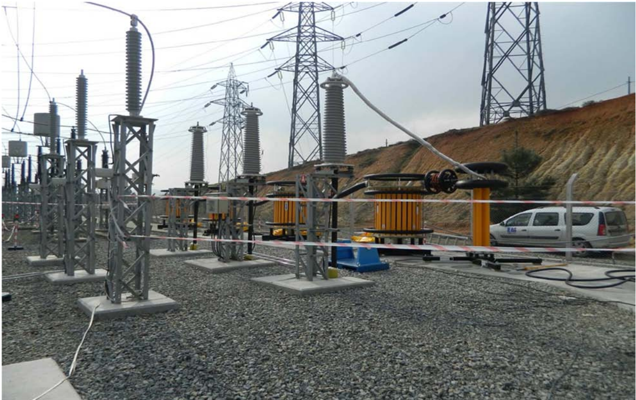
Figure 1. Reactors test assembly onsite in 4P connection
