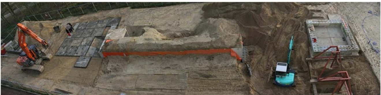
Fig. 1: Construction of the test site; in the middle tunnel elements and at right hand side termination supports
