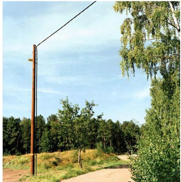
Fig.2. Cable coming up from the ground and continuing as aerial cable
